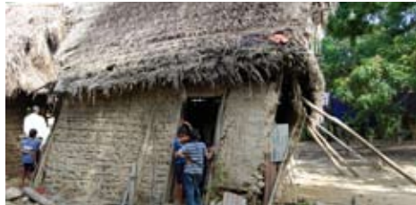
Families still living in storm damaged homes.
